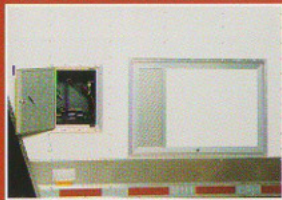
Exterior generator storage area and battery access compartment.
